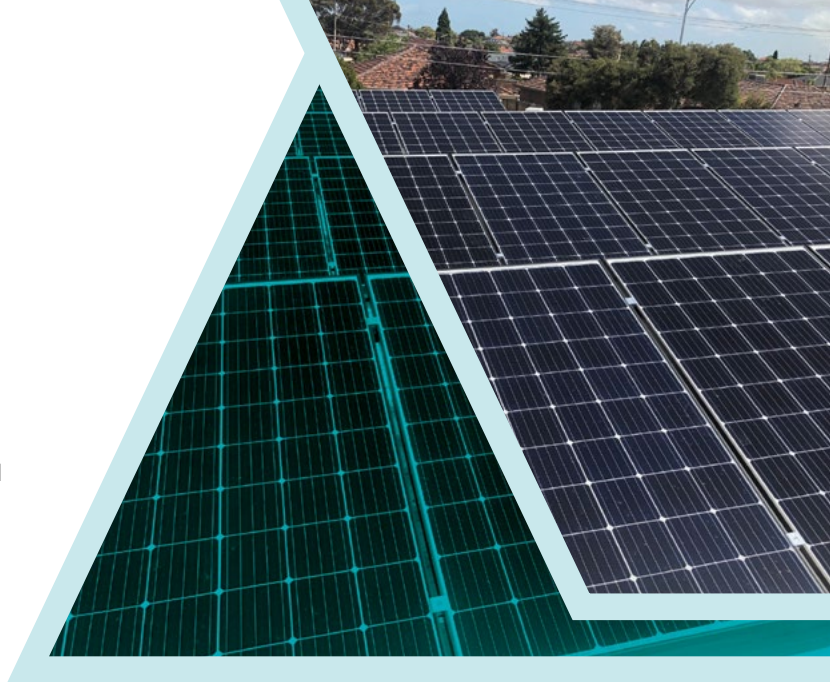
An installed PV system at Lalor Garden Primary School.
